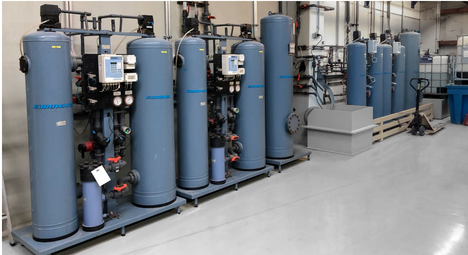
Multiple DI water production lines for pretreatment of light alloy wheels.
